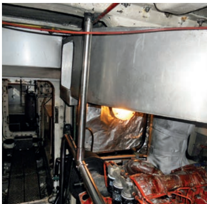
Old engine room ducting
