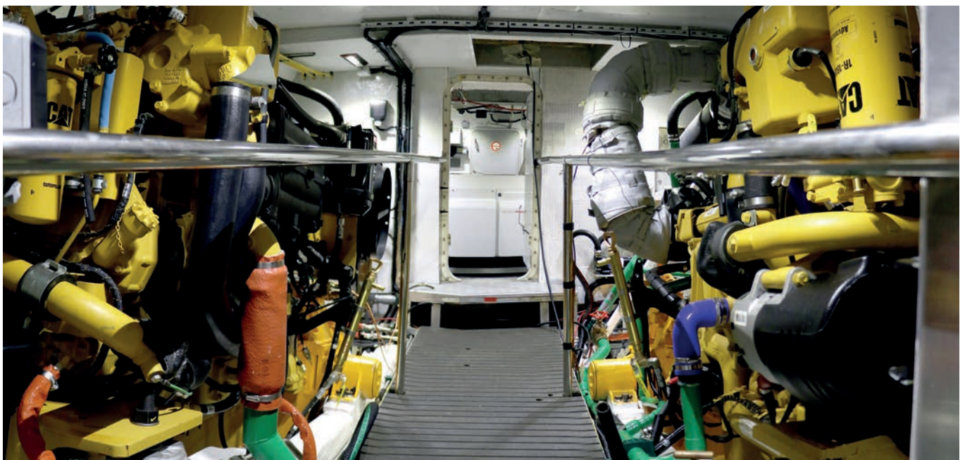
Installation of twin Caterpillar C18 810HP engines to a 60' stretched Arun MOD Police patrol boat
