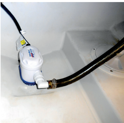
new bilge pump
