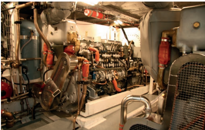
Refitted engine room
