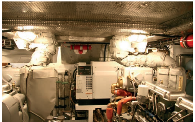
Refitted engine room
