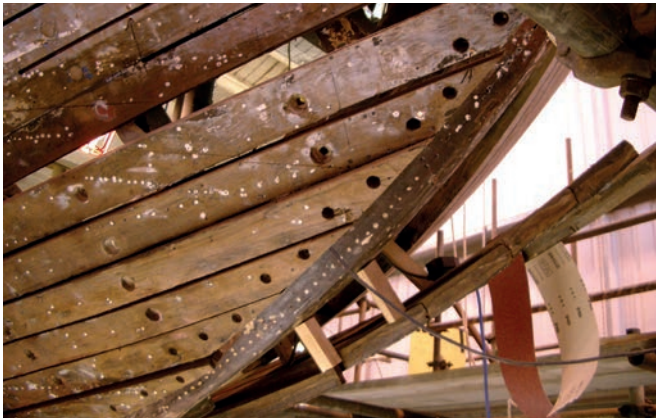
Original damage to stern
